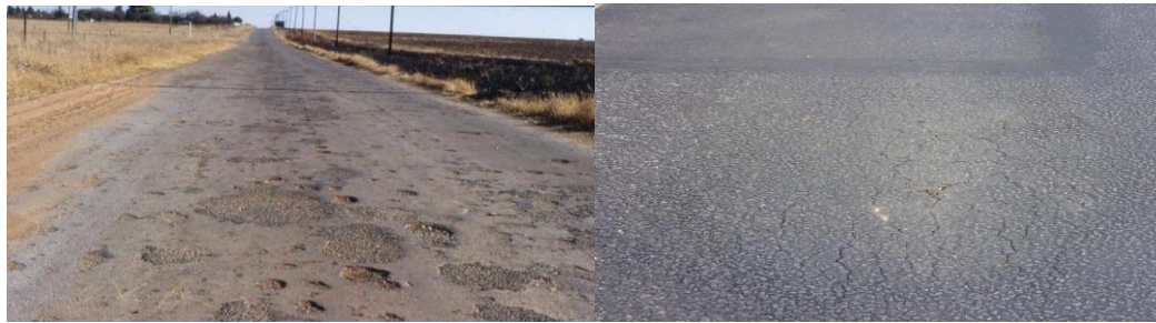
Fig 2. Development of potholes and fatigue cracking on a low-volume road with thin bituminous surfacing and insufficient preventative maintenance
